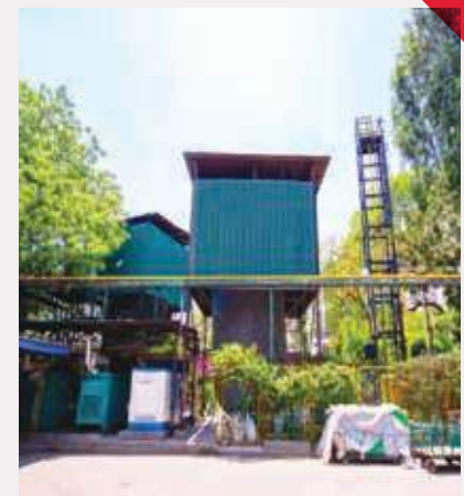
Biogas system, MIL Hapur
