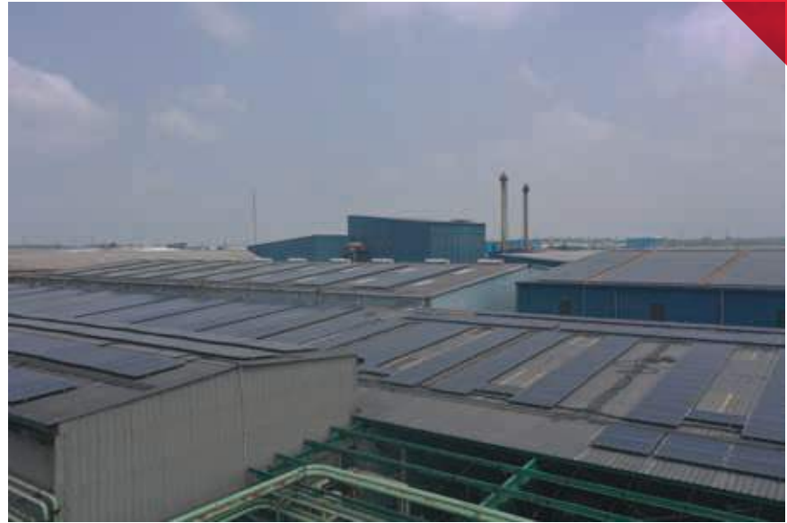
Rooftop Solar System MIL Rohad (H.R.)
