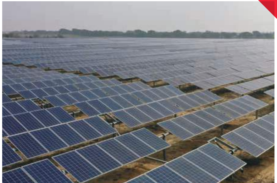
Groundmounted Solar System - Merino Rohad (H.R.)
