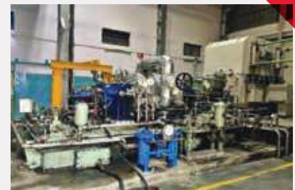
Biomass based Turbine, Hapur
